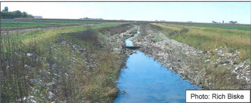
Figure18. Upstream end 1 week post September 2010 flood.
