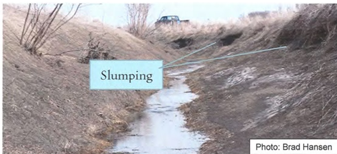
Figure 9. Portions of pre-construction ditch with slumping.
