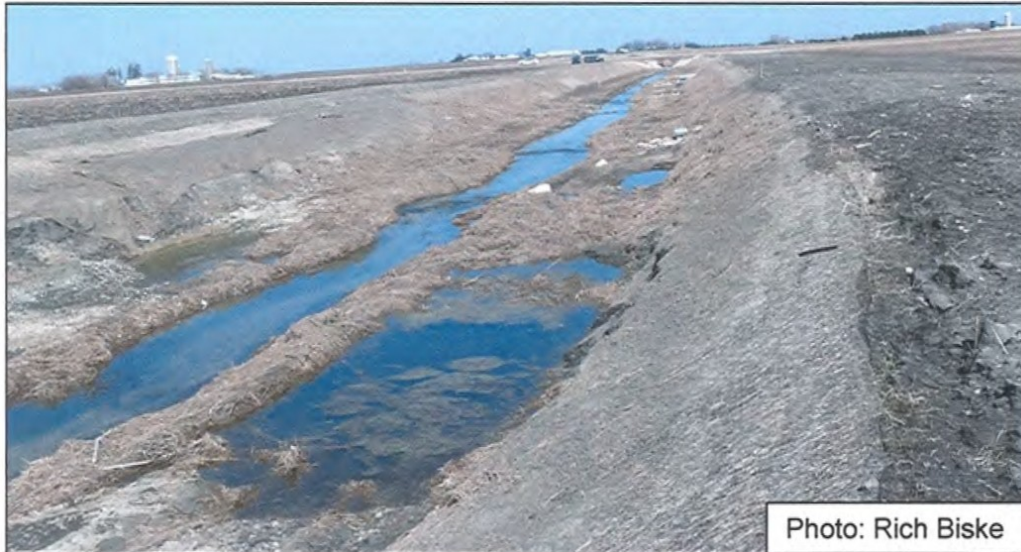
Figure 21. Bank failure on 2-stage ditch spring 2010.
